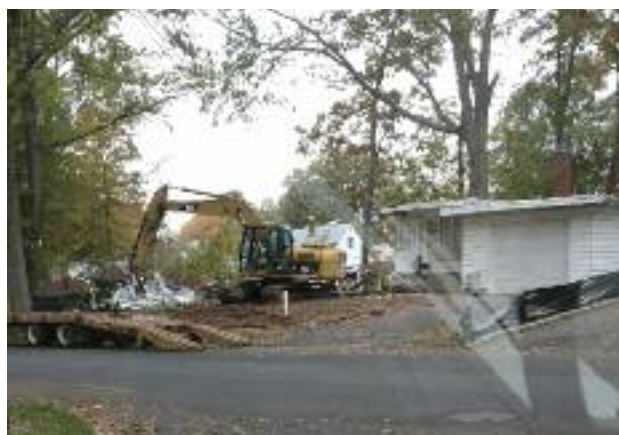
Minnie's home being demolished - and thanks to our ACO John DiStano, without Minnie trapped inside!
